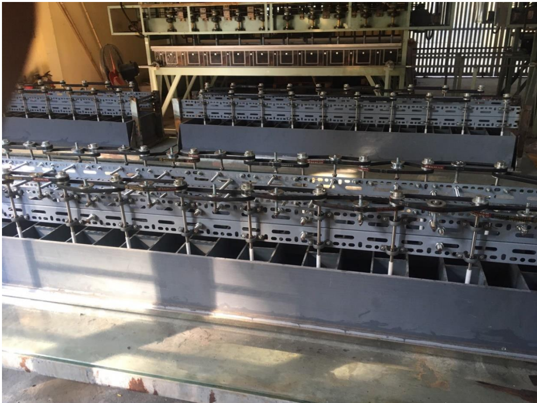
Fig. 5. The 20-stage mixer-settler system after finish.
